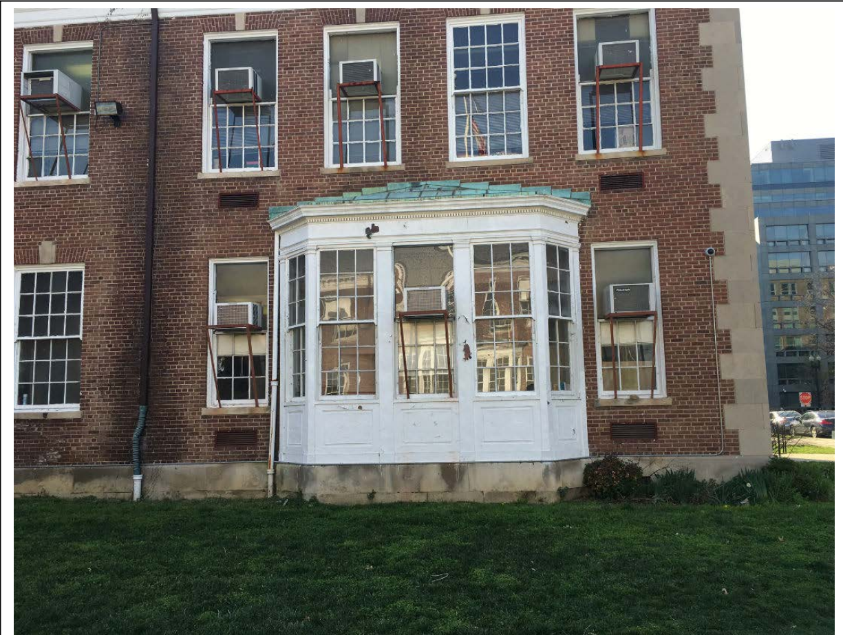
Peeling paint on front of house windows at Capitol Hill Montessori at Logan
